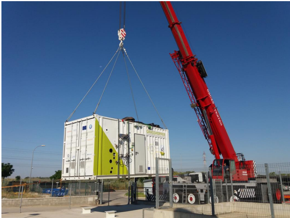
Figure 10 –Installation of the GRASSHOPPER pilot plant in the Abengoa’s testing facilities (port of Seville)
